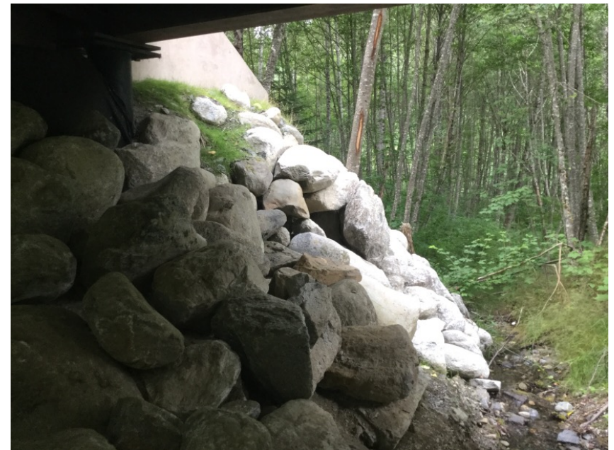
Oversteeped Left Embankment
