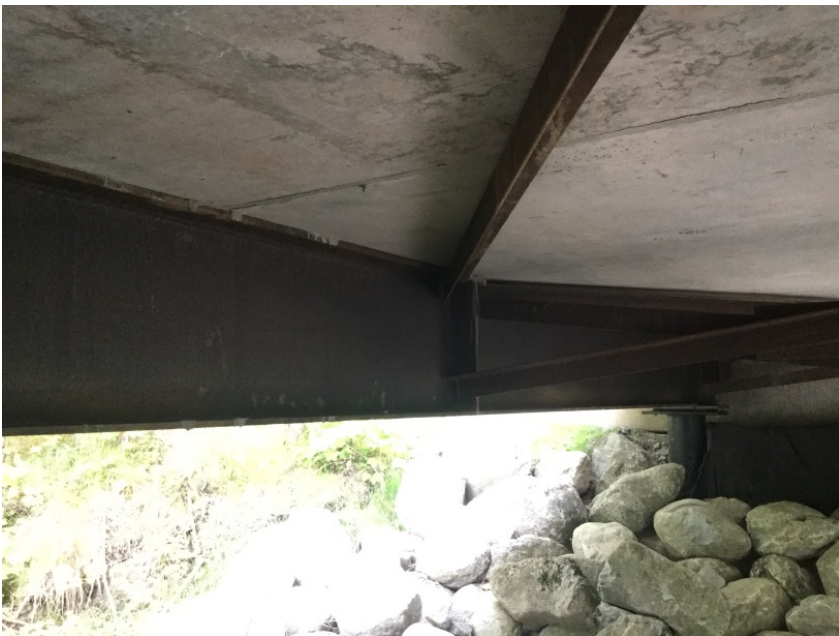
Girder and Bracing Condition
