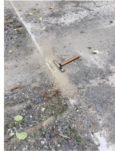
Spall in Wheel Track at Right Abutment Deck Edge
